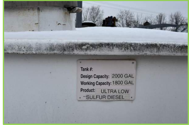
Circular diesel tank
