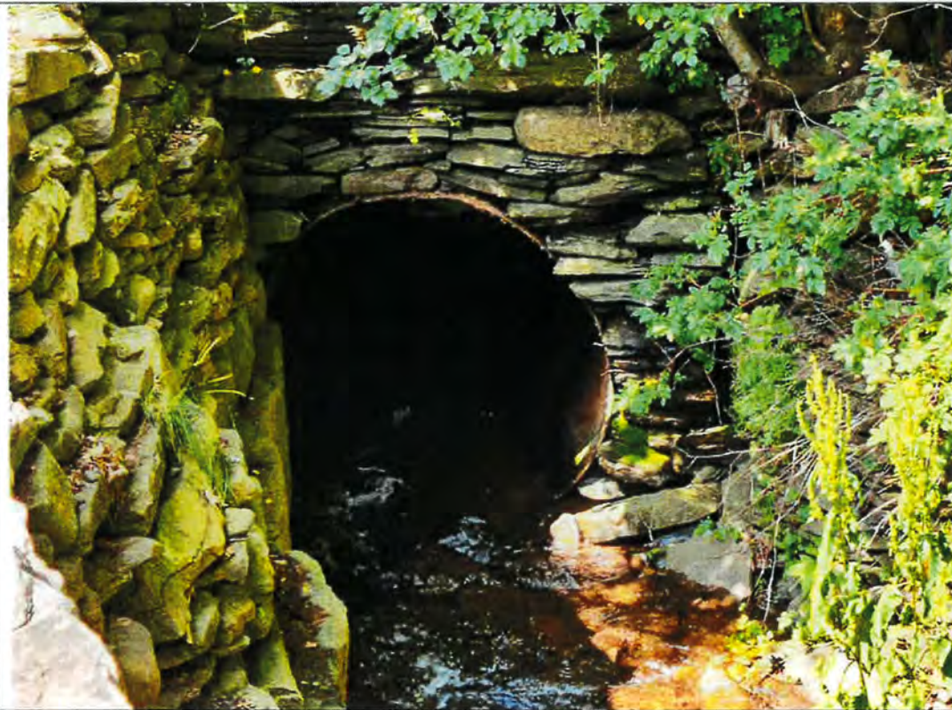
Photo 4: A closer view of the culvert inlet with the constricting opening. The wide stream channel narrows down to the metal boiler plate culvert inlet.
