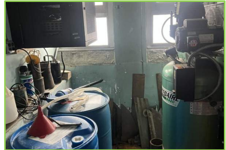
Equipment room - Diesel exhaust fluid blue containers
