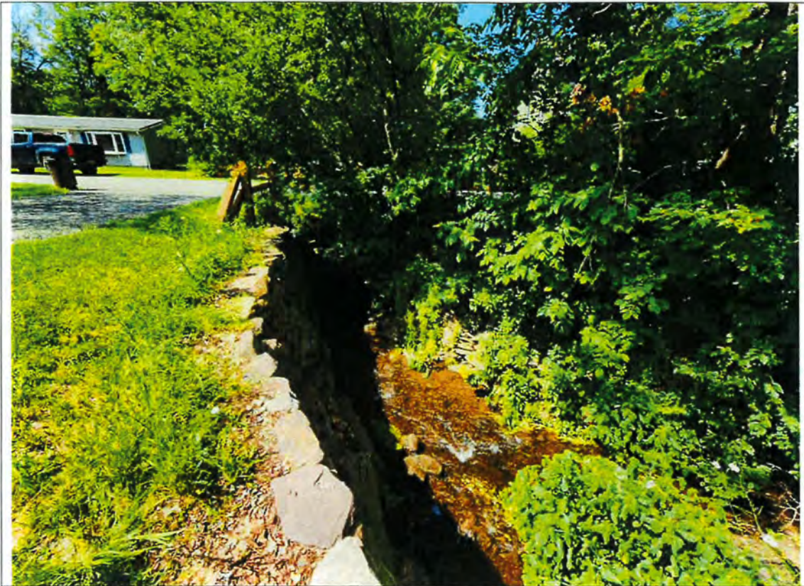
Photo 3: Looking downstream at the culvert inlet. Note the constriction of the stacked rock wall on both streambanks.
