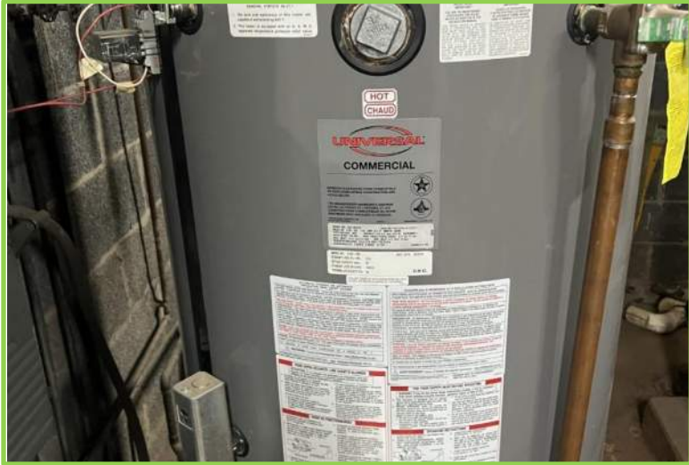
Boiler room tank
