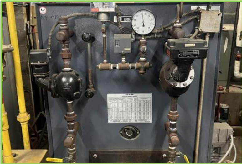
Boiler room pressure gauge
