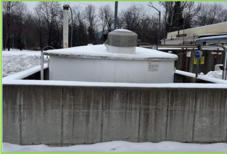
Circular diesel tank
