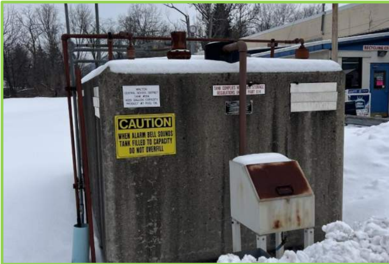
Rectangular tank (not used)
