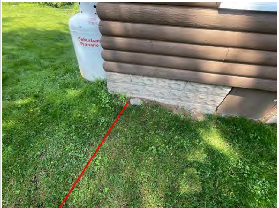
Brown House: Location of 3/4" water line to blue house noted
