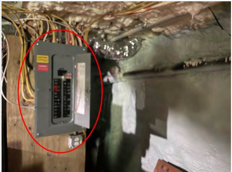
Red House: Electrical panel noted
