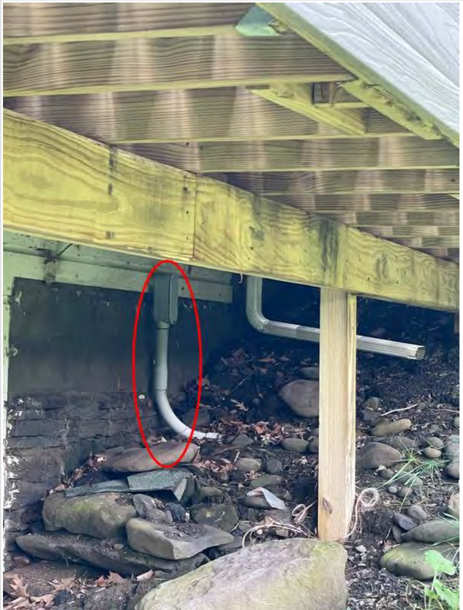
Red House: Electrical main noted
