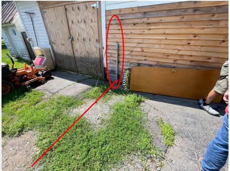
Caretaker House: electrical line btw from white house noted
